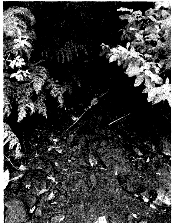
RIPRAP AND BANK FAILURE STA. 2+00 APPROX.
