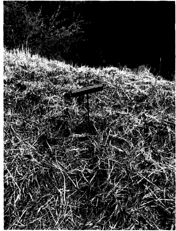
RODENT HOLE WITH PROBE PENETRATION 2.5-3 FEET
