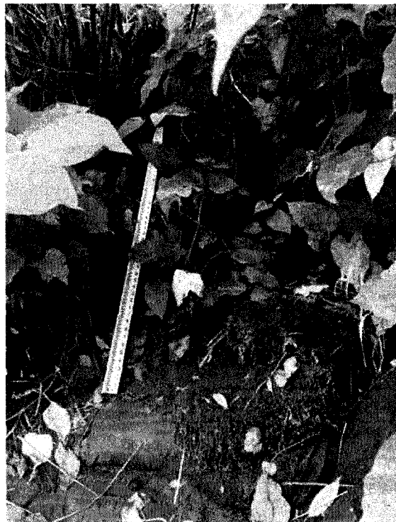
BANK FAILURE ABOVE SANDBAGS STA. 1+50
