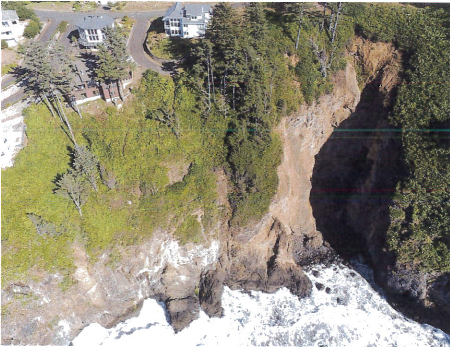
Photo 4 - Oblique aerial photograph of the bluff in the area of the site.
