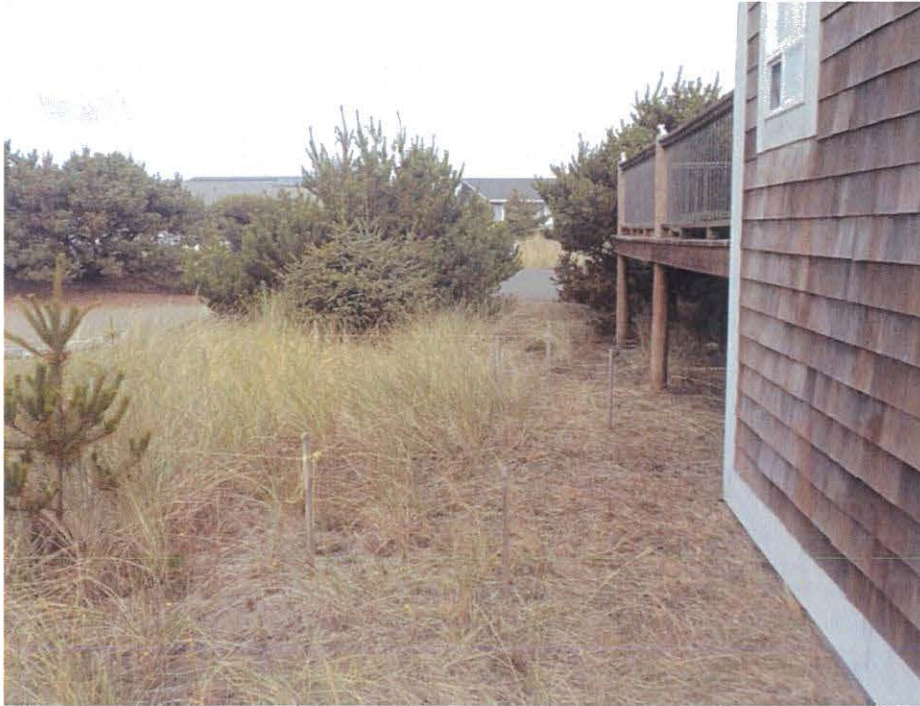
Photo 3 – View of the existing deck at the northwest corner of the house and the location of the proposed new elevated deck.
