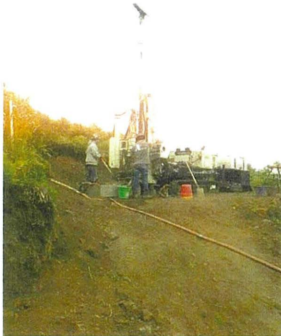
Photo 11 – View of the mud rotary drill rig set up at Boring B-1 (2019).
