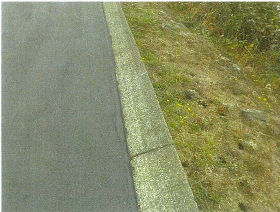
Photo 16 – View of the recent pavement surface coating along the northern portion of the site. (2022).
