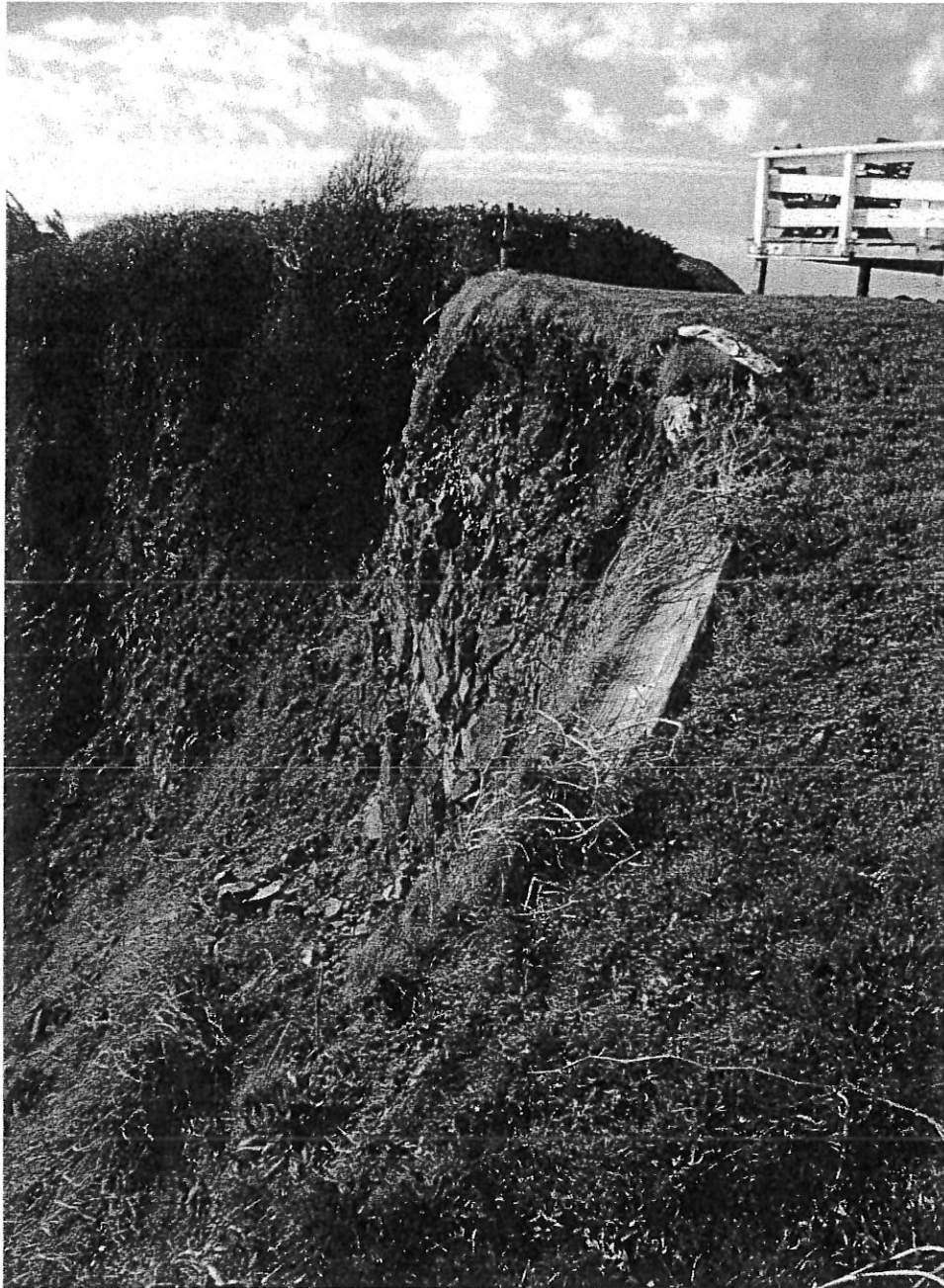
Photo 3 - Looking northwest along the failing upper edge of the southern bluff slope.
