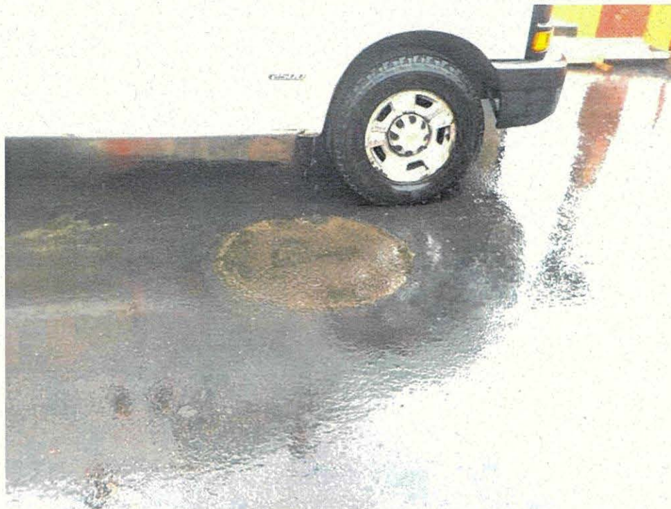
Photo 8 – Close-up view of a manhole near the site indicating the potential presence of buried private utilities and installations.
