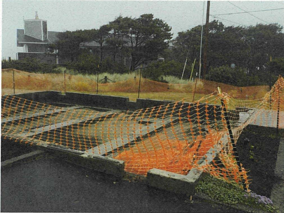
Photo 1 – View of the foundation of the previous house at the site after demolition.
