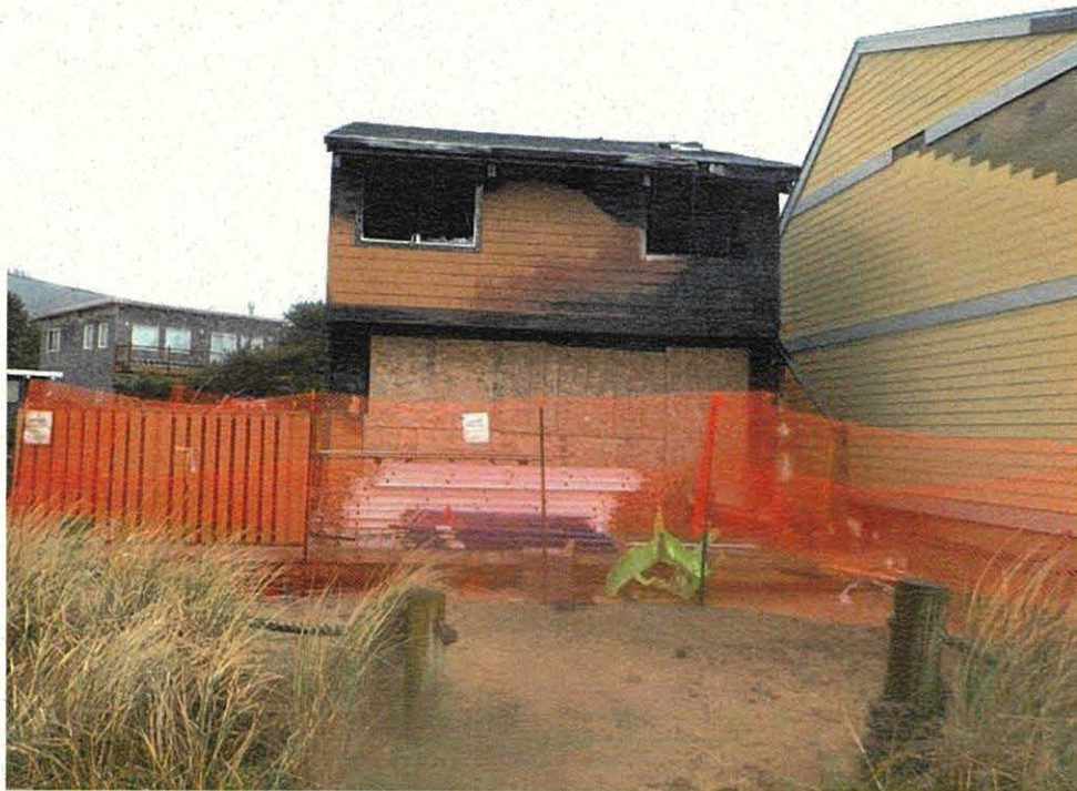
Photo 2 – Southeasterly view of the subject site occupied by the existing fire-damaged residential building.
