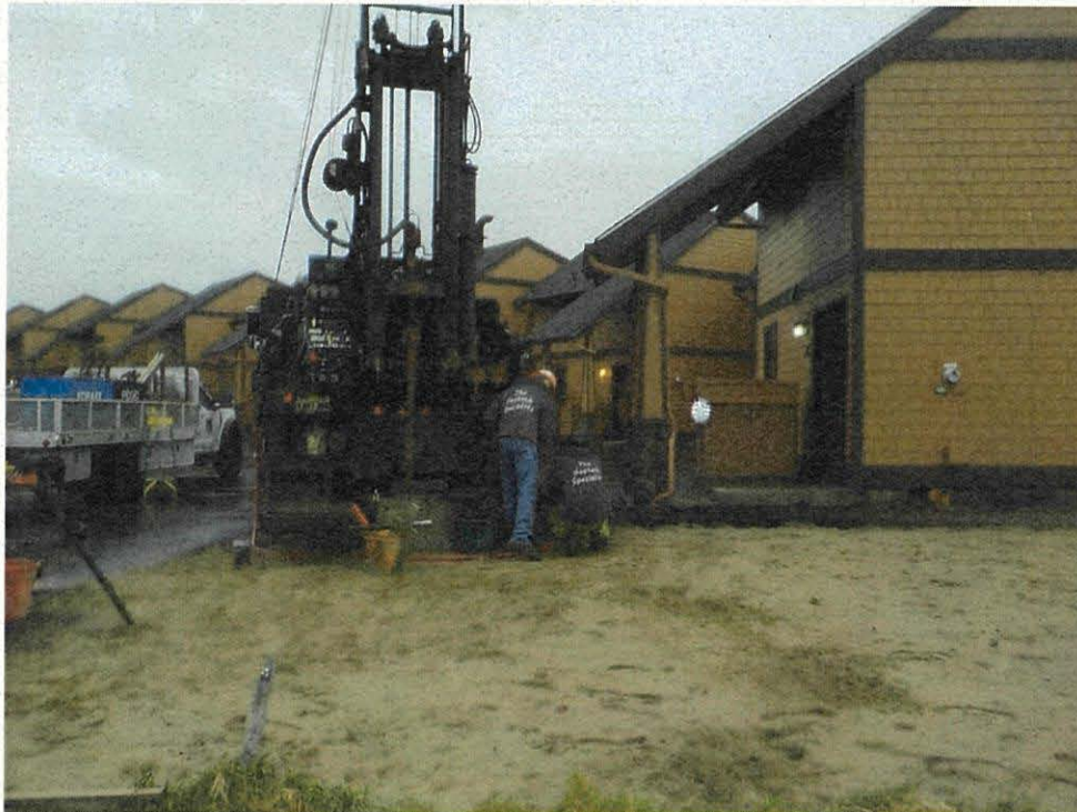
Photo 2 – View of the drill rig set up at the location of Boring B-1.
