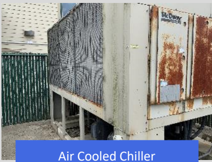
Air Cooled Chiller
