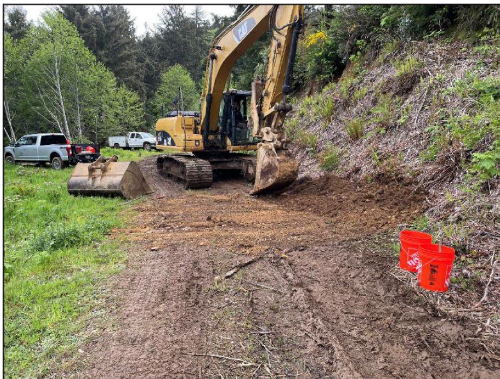
Photo 2: Photo looking northeast along the existing road before the creek. Note that the existing road cut has an oversteepened slope.
