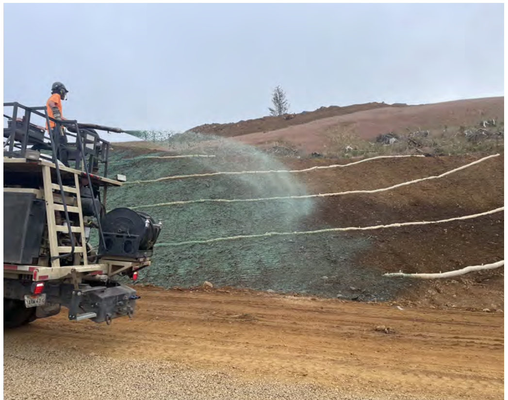
View of seeding of roadway embankments behind the recently completed MSE walls.
