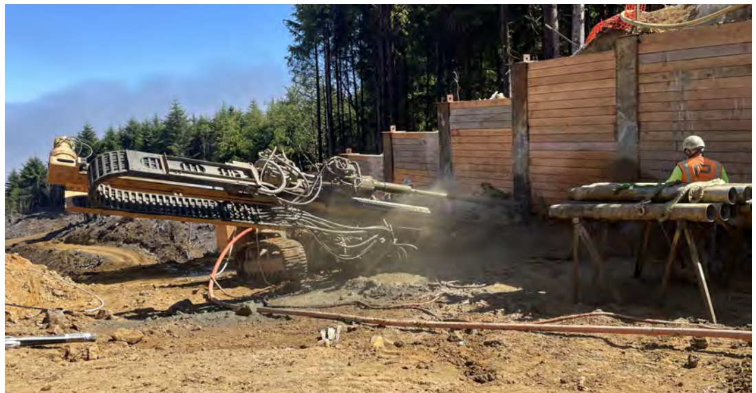
View of horizontal drilling at soldier pile wall during ground anchor installation.
