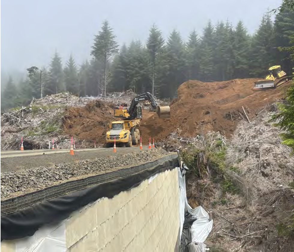
View of roadway excavation north of Coleman Creek at the geofoam wall.
