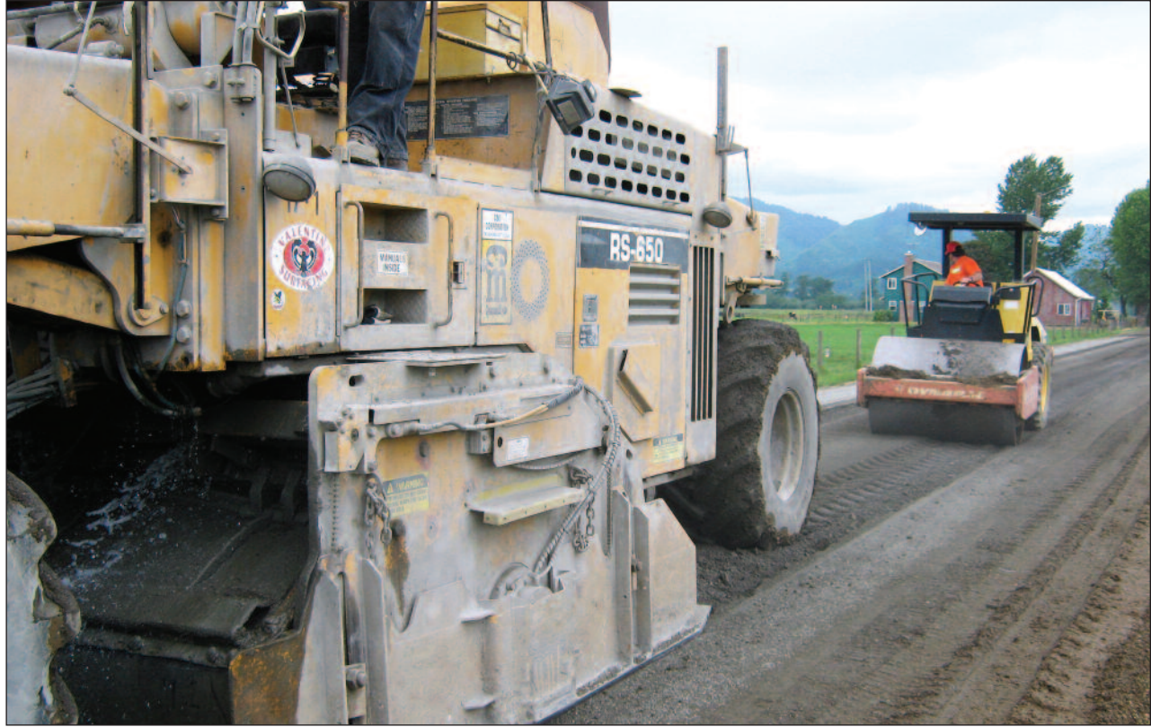
Grinding machine recycles a section of McCormick Loop during a resurfacing project.
